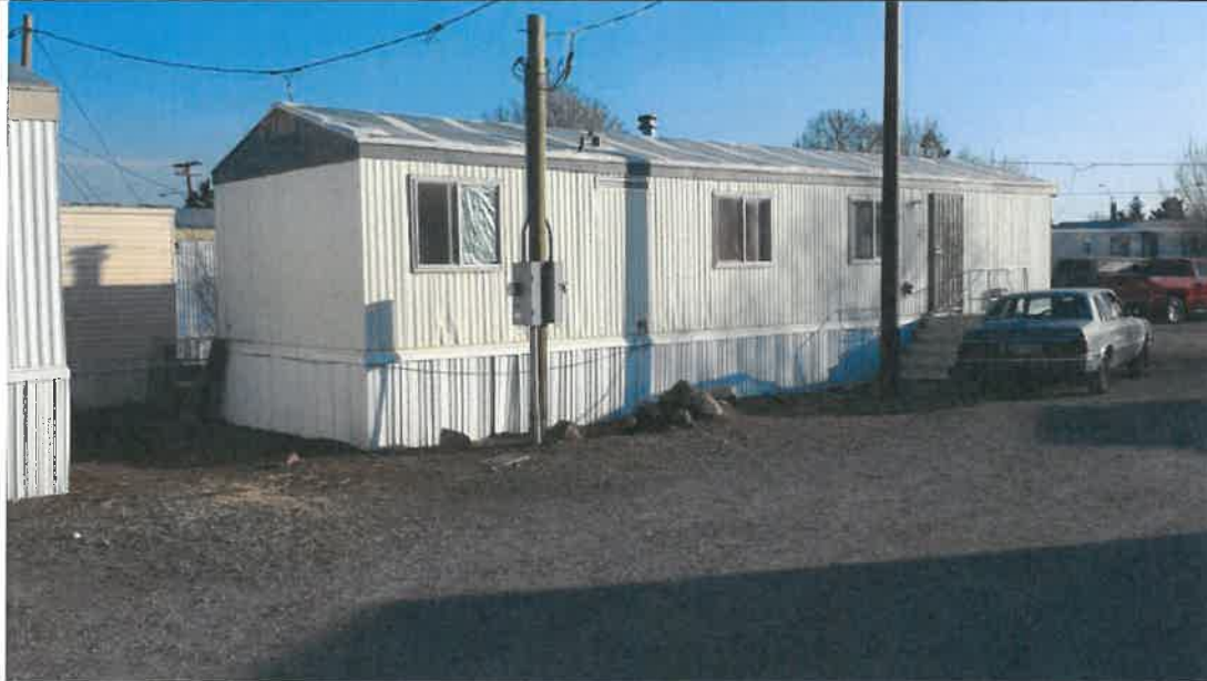
Photo 1 of 3 taken 11-18-14: Looking southeast at north and west sides of home. Electrical meter is detached and service is above the RFE. Small box attached to building behind car and detached stairs is a mail drop off box. Skirting is flexible vinyl.
