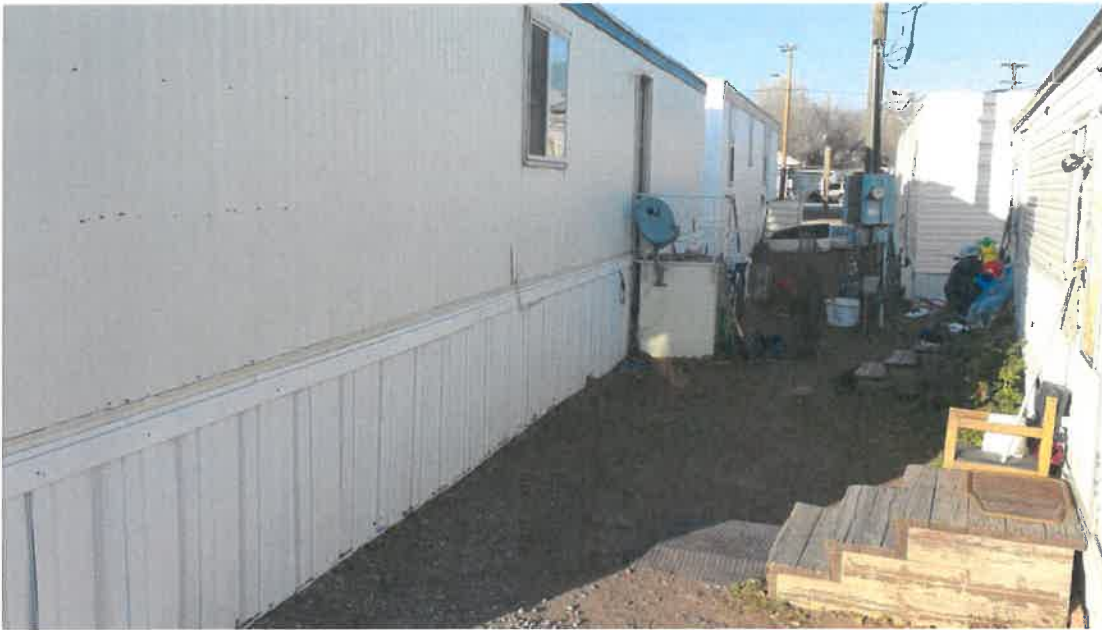
Photo 3 of 3 taken 11-18-14: Looking north-northwest at east side of home. No electrical or mechanical equipment is attached to the building. The satellite dish is not electrical, and is attached to detached stairs.
