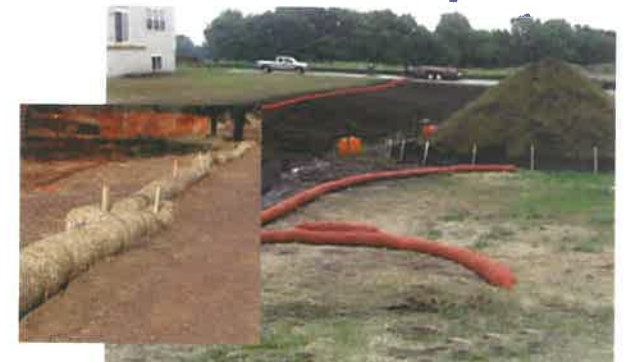
Straw wattles or silt fence works well as perimeter sediment control AND as stackpile protection.
