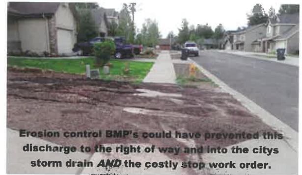
This project was flooded due to construction site runoff of sediment and debris.
