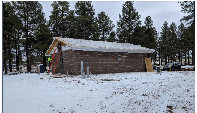
The new pumphouse disinfects the water prior to entering the distribution system.
