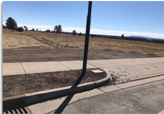
Unnecessary curb cut provides unauthorized vehicle access to McMillan Mesa identified for removal.
