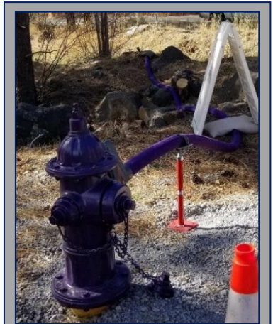
Purple hydrant pumps Class A+ reclaimed water from Buffalo Park tank.
